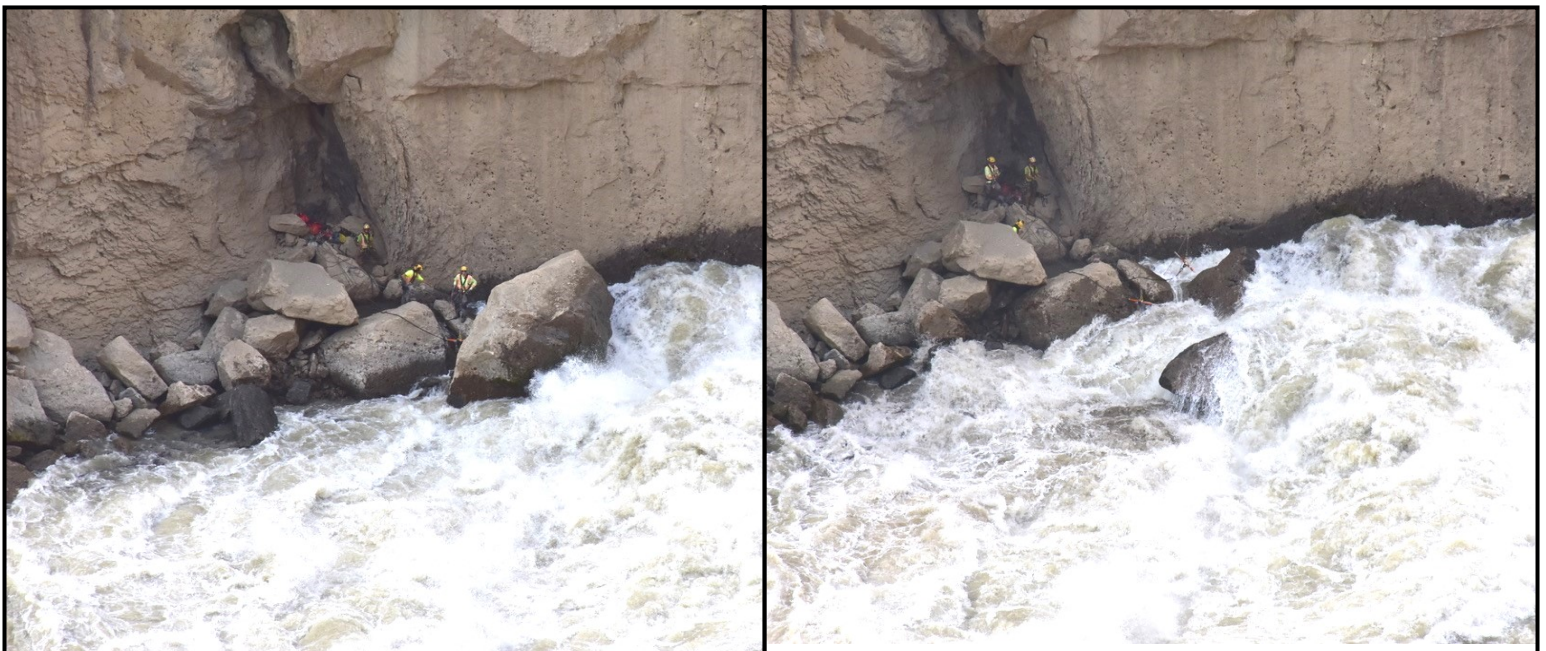
Before and after pictures of a rock that was manipulated by the rock scaling crew.
